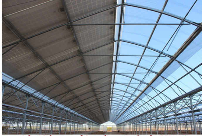
Solar PV integrated Greenhouse Project by SOLTEC
